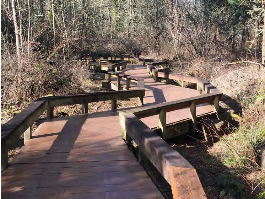
Irregular jogs and uneven elevation changes
