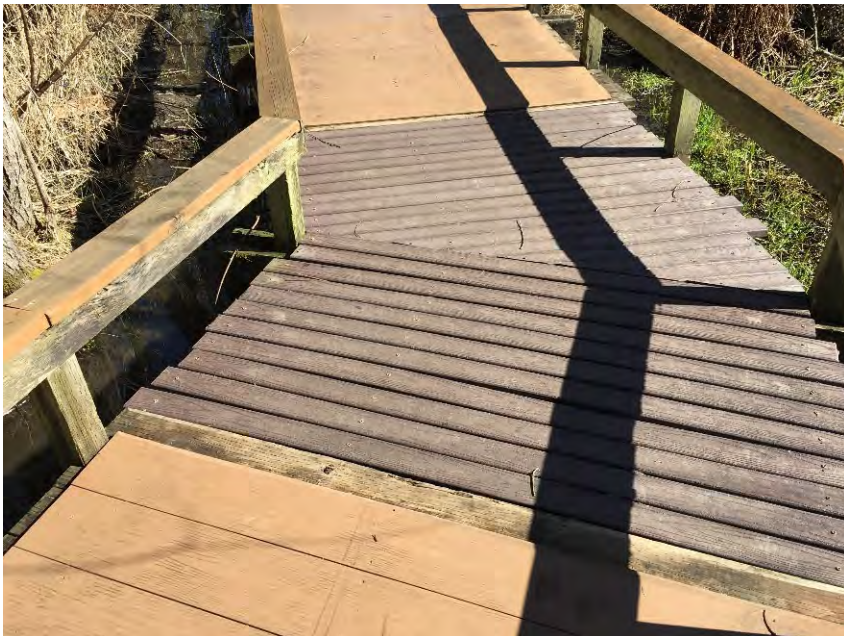
Worn and inconsistent surfacing
